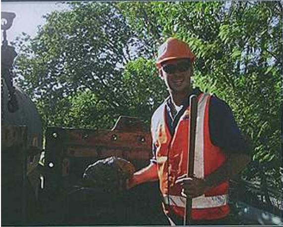
An example of material obtained from the obstruction strainer.
